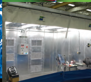
ATI Environmental Control Booth
